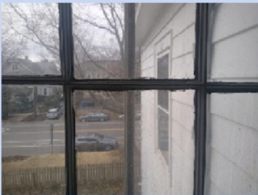
Misaligned mullions and structural decay
