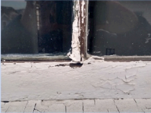
Exterior weathering and rot to sash
