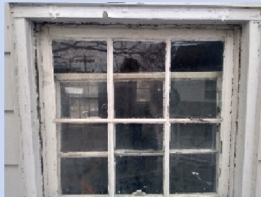
Overall weathering and rot to sash and frame
