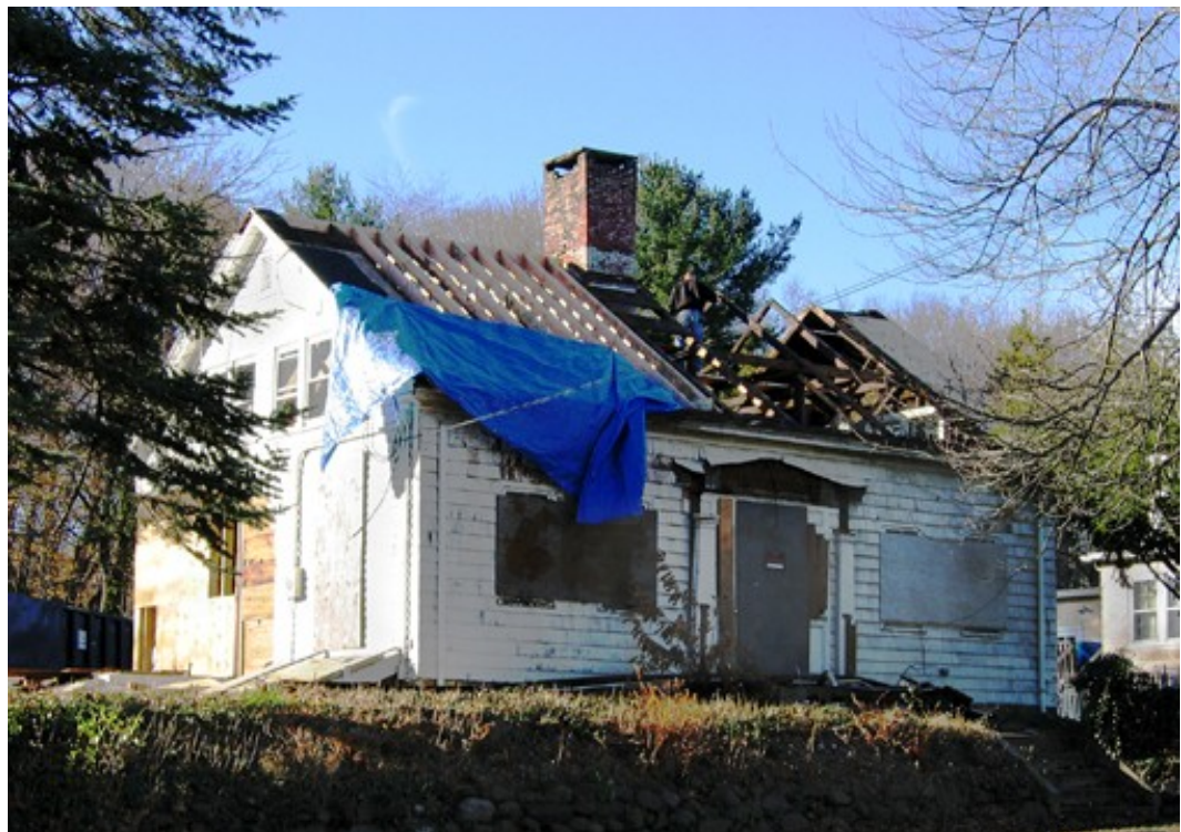
324 Townsend Avenue. This colonial era building is being structurally reinforced and secured for future restoration. The Historic District Commission worked with the Parks Department on an historic structures assessment to document the essential elements of the building and to identify the historic core for preservation.
