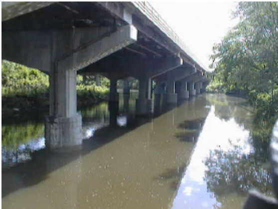
View from State Street looking south at the elevated roadway section of I-91 over the Mill River.
