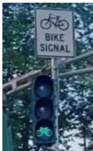
Figure 2.13 Bicycle Traffic Signal Wall Street at Church
