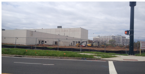
Construction is already underway to convert the former New Haven Register building at 40 Long Wharf Drive to a 200,000 square foot Jordan’s Furniture store featuring both retail and family entertainment opportunities.
