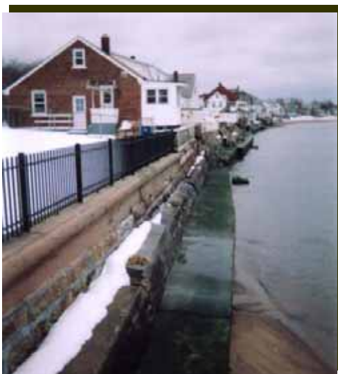
Pardee seawall and privately-owned seawalls at low tide with very little beach material
