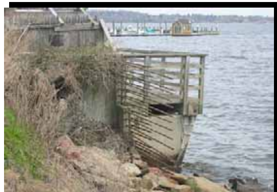
Incomplete public access at Harbor Landing
