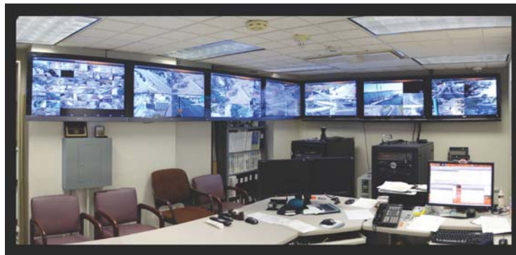
Signal Division Control Center for Traffic Signal Intersection Management
